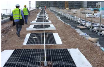
Fall protection is ensured both with guardrails and with rails including a mobile attachment point.
