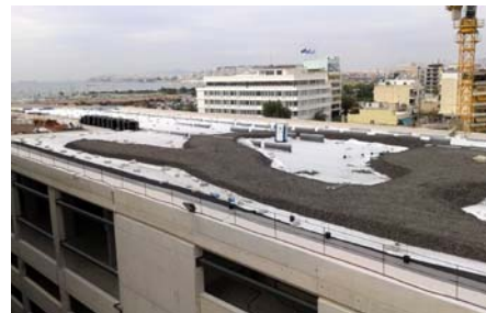
Glass foam gravel was used in some areas in order to achieve a higher total build-up.
